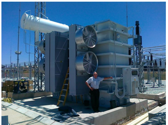
Picture: 120 MVA 132/66/11 kV Trf:
