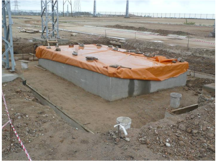
Picture: 120 MVA Auto Trf Plinth
