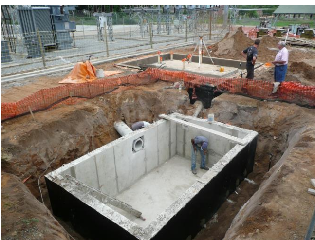
Picture: Trf bund wall and oil sump
