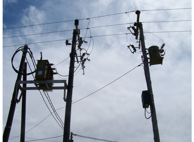
Picture: Connection to the 11kV network
