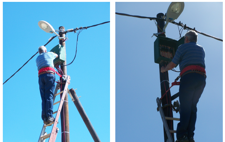
Picture: Installation inspected by BDE
