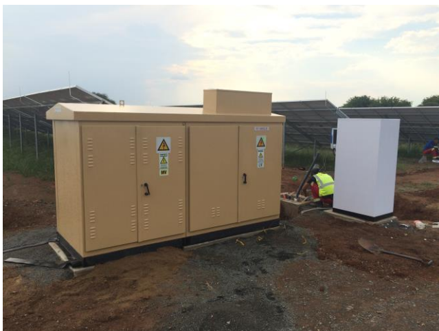
Picture: 400/11000 V step-up transformer:
